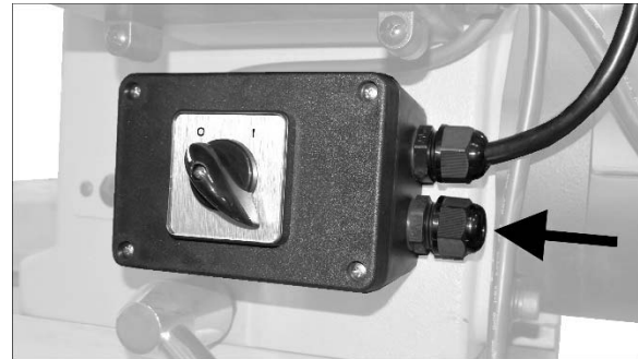
Figure 7-1: main switch box
